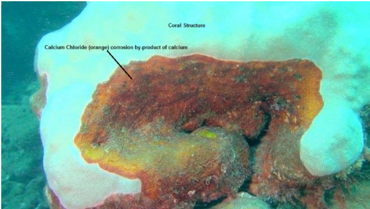
Figure 5: It appears the Calcium carbonate reef structure is corroding to oxides and salts beneath radar stations in Kaua, HI. Photo Compliment by Terry Lilley, Kauai, HI. Calcium Chloride precipitate is orange.
